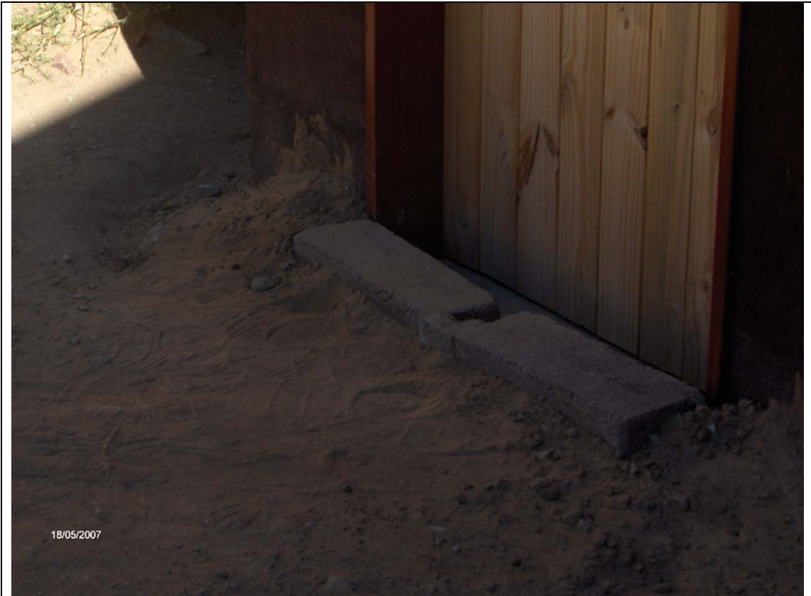
Pic4: Intervention by beneficiaries against storm water, Surface bed below ground level
