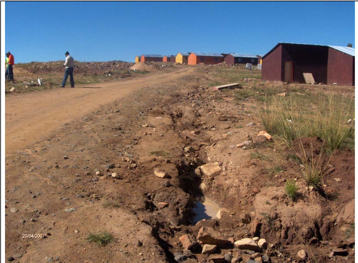
Pic6: Storm water damage
