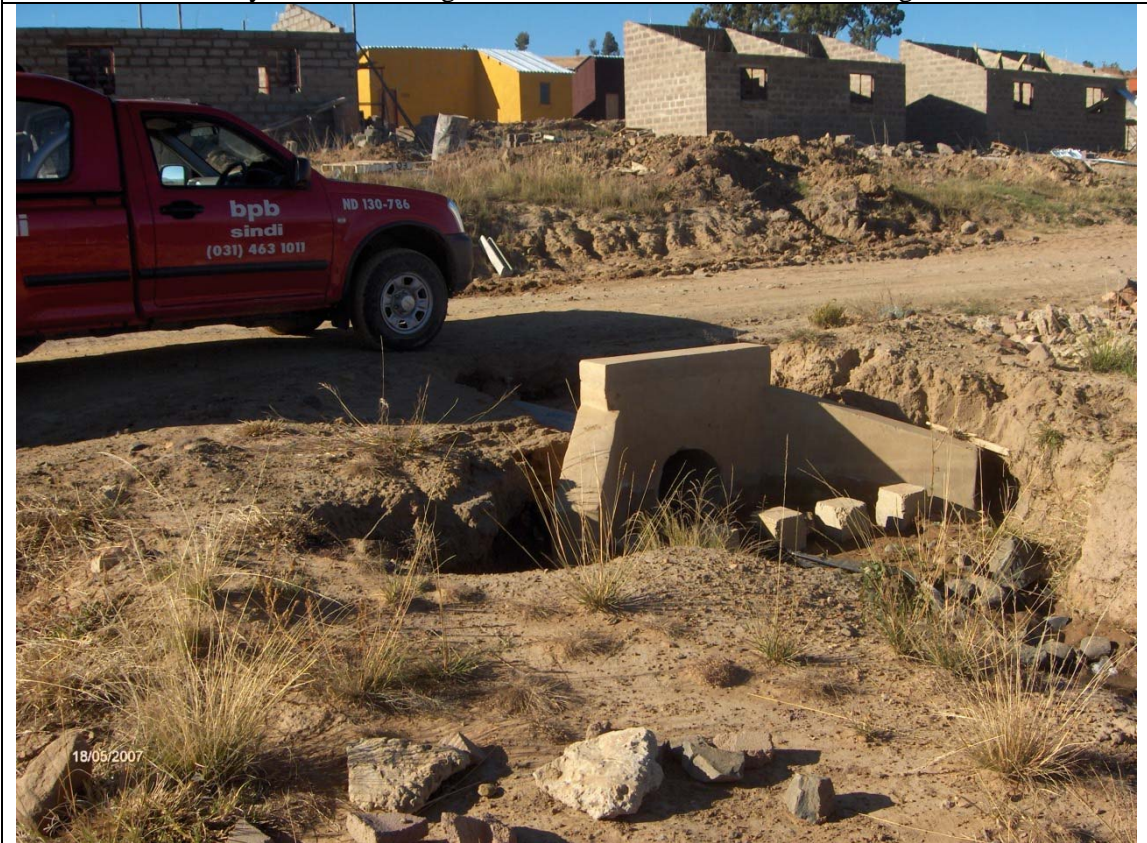
Pic5: Storm water damage
